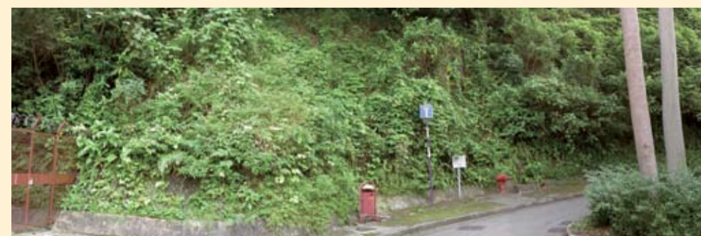
九十年代在崇基職員宿舍附近蓋滿灰泥護面的斜坡（上圖）；同一斜坡的現貌（下圖）。 Before: a slope covered with chunam plaster near Chung Chi staff quarters in the 1990s (top) After: the same slope now (above)
