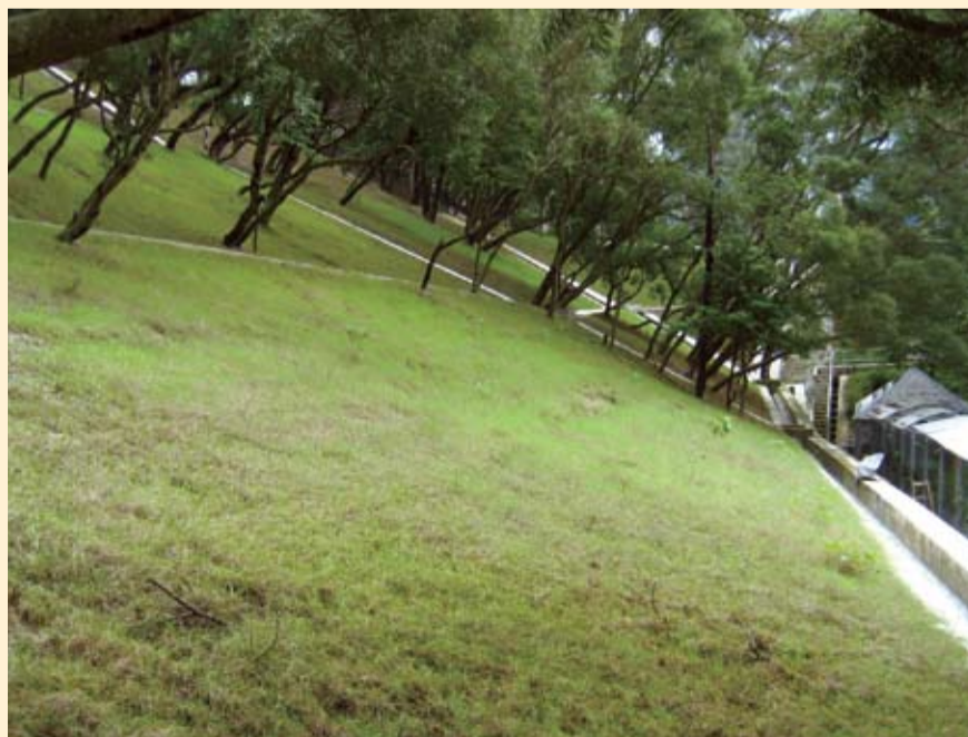
在邵逸夫人樓附近的回填坡，是藉挖坑種植來鞏固的。這種方法可盡量減少移植樹木，部分過程須用人手處理，耗時較長。 A more time-consuming method of stabilization—trench excavation—was used to stabilize this fill-slope near the Lady Shaw Building so tree removal can be minimized. Part of the procedure was carried out manually.
